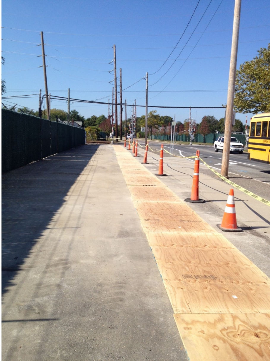
Covered trench and work zone at 60/66 North Clinton Avenue adjacent to Clinton Avenue
